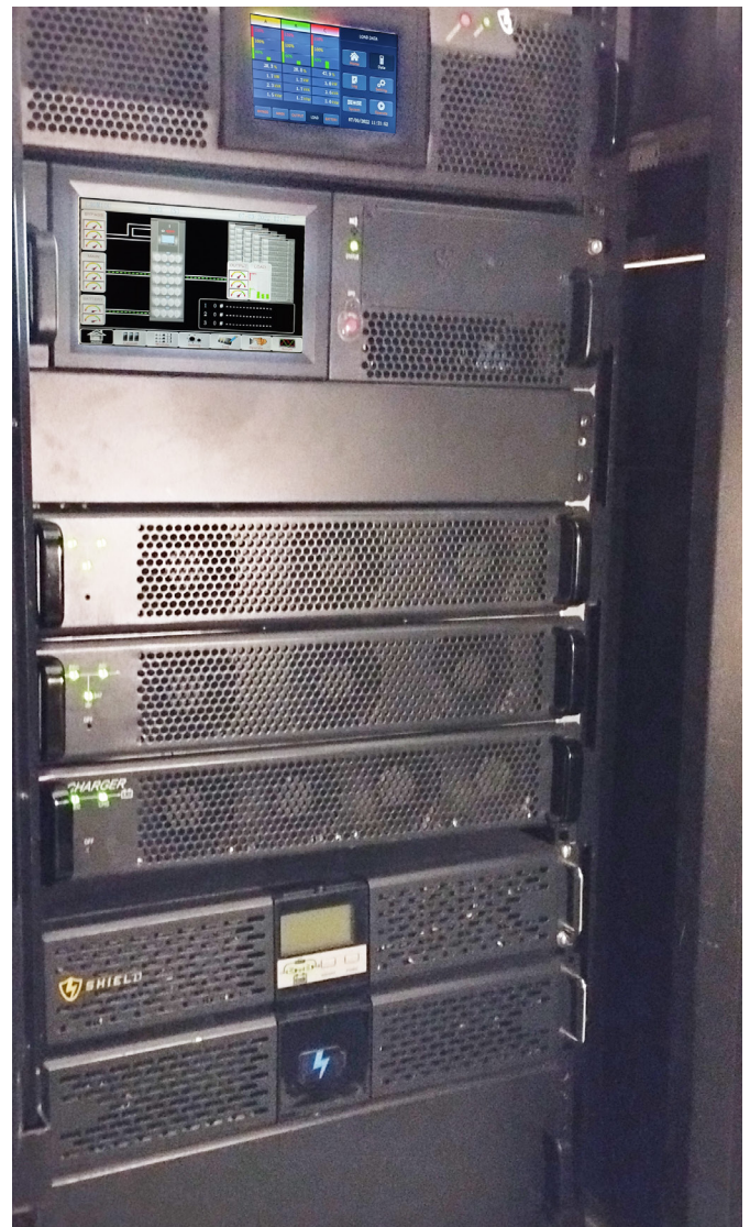
The UPS installation at Techno Brain with a supercharger
