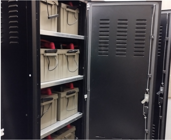
External battery racks that required for a longer runtime
